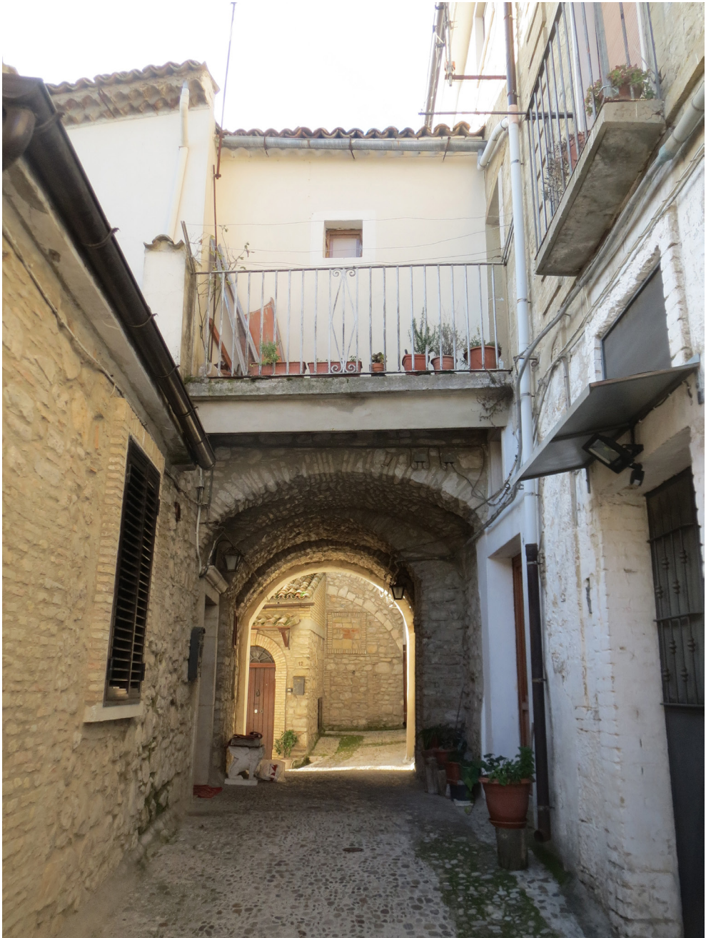
Fig. 9. Sant'Agata di Puglia (FG). View of a connecting vault between two facing blocks set on different contour levels. An effective anti-seismic measure but one which has undergone inappropriate additions (photo by the author)
